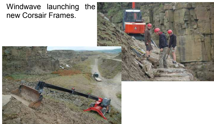
Construction work in the quarries putting the trails and paths in place.
